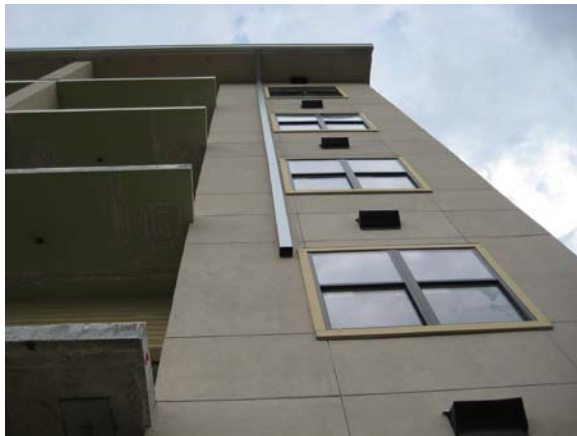
Vol. 4 – bldg 16 west elevation downspout (SW corner) not placed correctly
