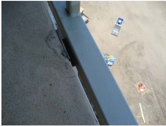
Spalled concrete at balcony edge / damage to finishes not touched-up prior to screen installation (building 17)
