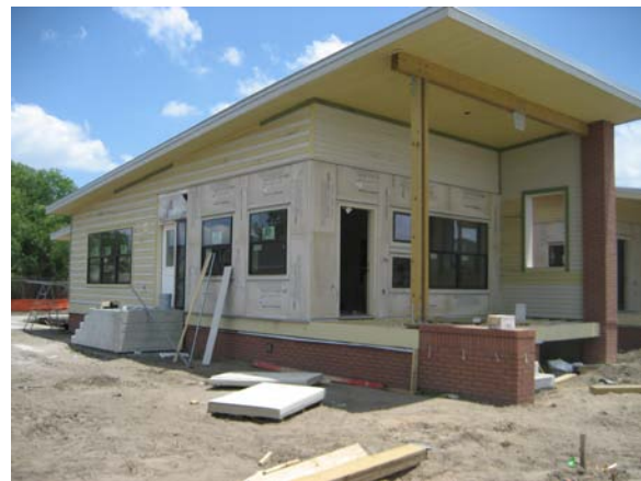
Hardi siding does not appear to be primed on white boards
