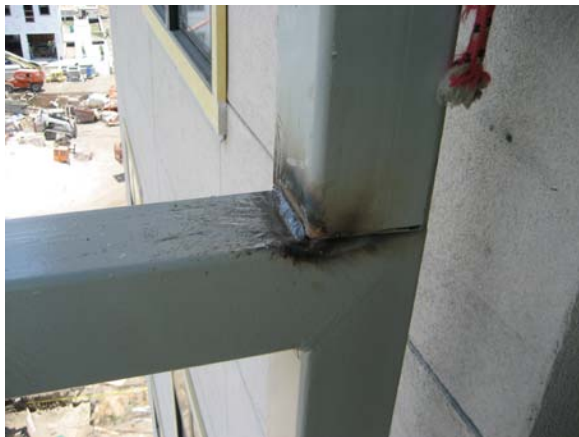
Repairs to galvanizing/finishes required at field welded connections
