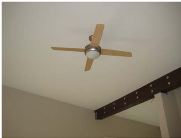
Ceiling fans in high-ceiling spaces are required to have longer stems for proper circulation and maintenance
