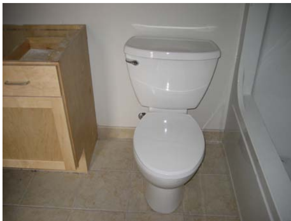
Toilet installation not level, typical condition observed
