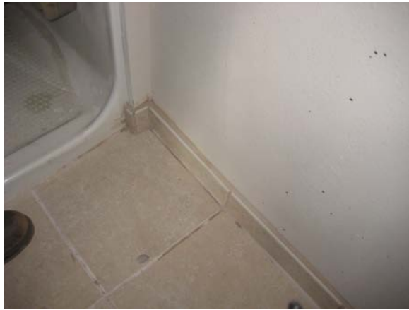
Vol. 4 – grout joint between base and wall too wide, rejected.
