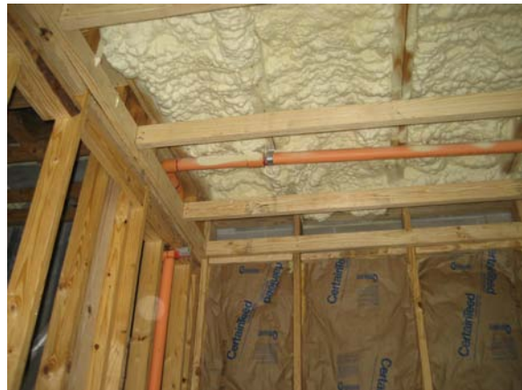
Lowered ceiling in volume 3 stairwells – not authorized.
