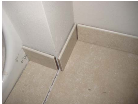
Vol. 4 – wall base joint too wide.
