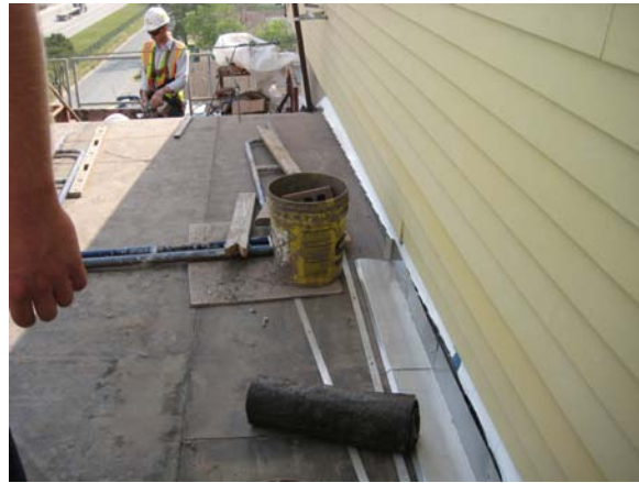
Volume 4 – Through-wall flashing height must be raised to meet or exceed contract document requirements
