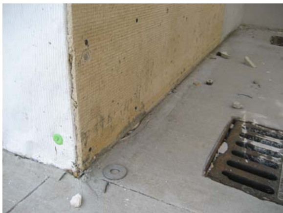
Volume 3 – typical wall condition. Cement board too tight against concrete, no flashing installed
