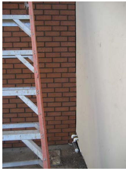
Volume 3 – joint between brick/stucco inconsistent and too tight in some areas for sealant.
