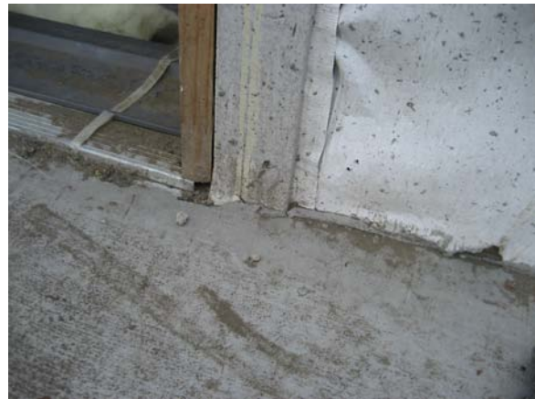
Volume 3 – entry door condition. Trim too tight against concrete
