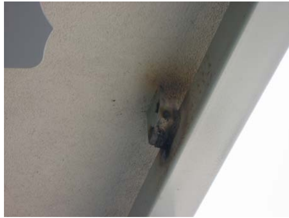
Unacceptable connection condition at soffit, building 17
