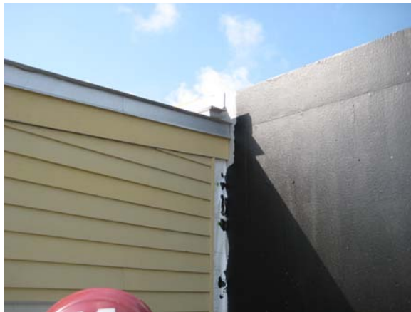
Volume 4 – flashing condition between framed wall and shear wall must be addressed prior to installation of brick.
