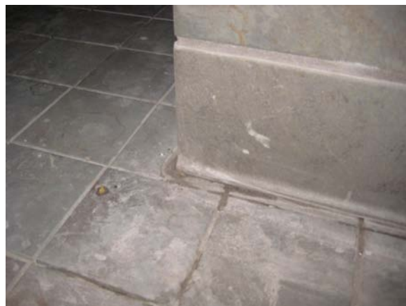
Incorrectly installed cove tile base at bldg 17 toilet rooms
