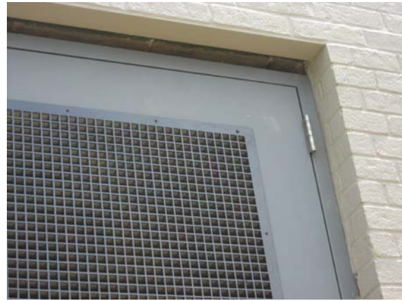
Frame head at electrical building door not correct
