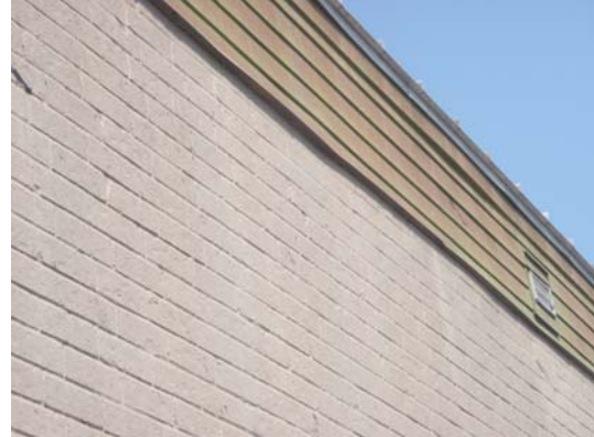
2 Entry building scorched
