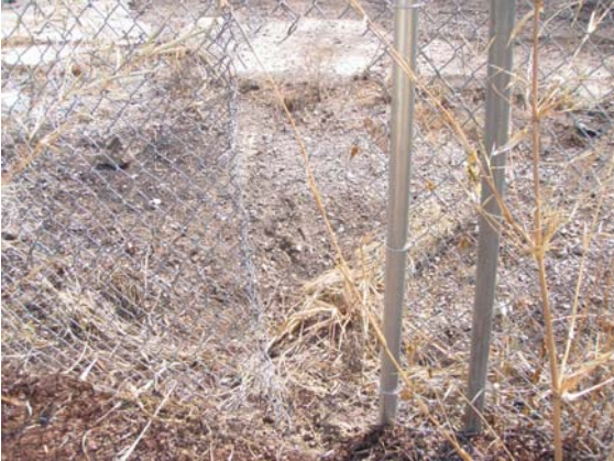
5 Hole cut in fence for fire dept access
