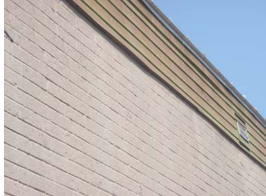
2 Entergy building scorched
