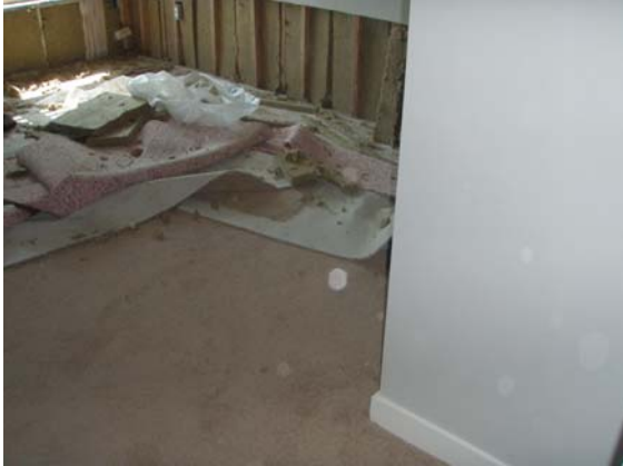
5 Carpet pulled back in building #2.
