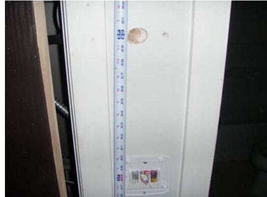
4 T-stats lowered to meet FHAA
