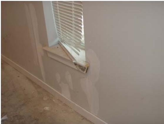
5 Probable mold growth in need of remediation
