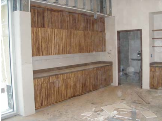
3 Cabinets in place in the Activity Center
