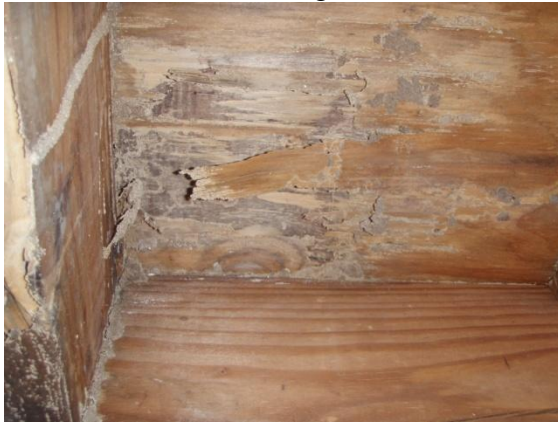
5 Probable termite damages
