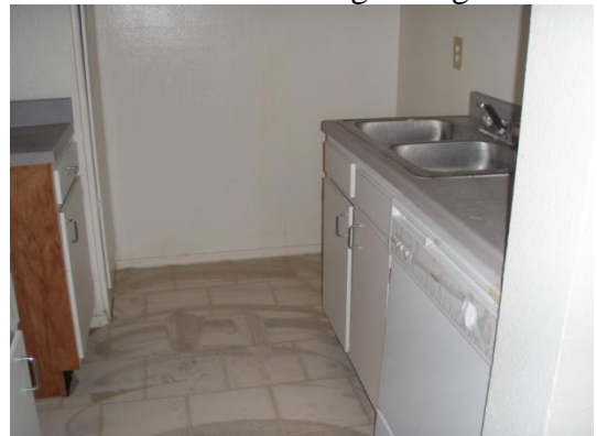
8 Outdated, inefficient appliances along with deteriorated flooring throughout.
