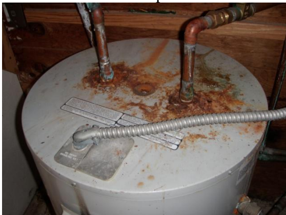
7 Water heaters in disrepair.
