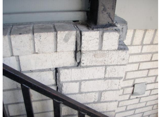
4 Evidence of structural failure.
