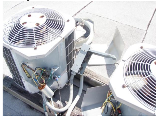
6 Inefficient HVACs also pose a danger due to possible vandalism.
