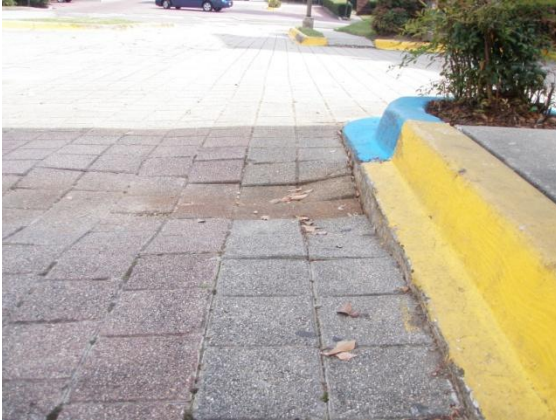
3 Failures within driveways and parking.
