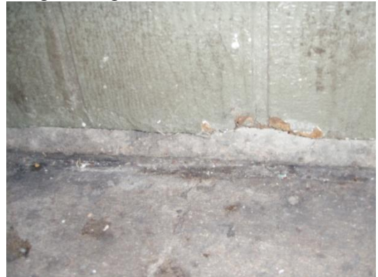
4 Signs of age and deterioration.
