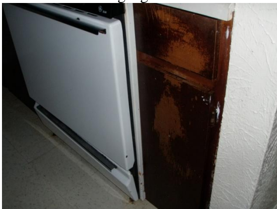
7 Cabinets showing signs of deterioration.
