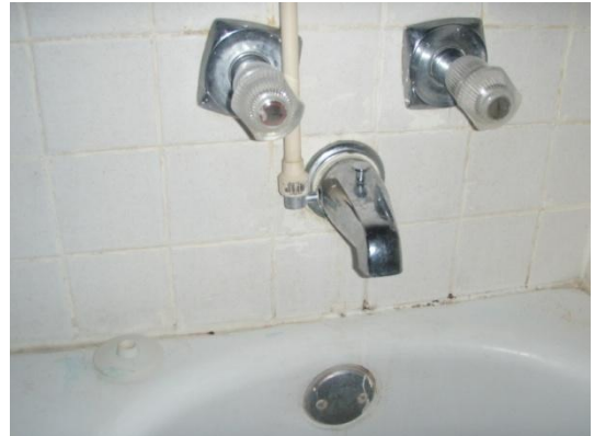
6 Bathroom needs rehab.
