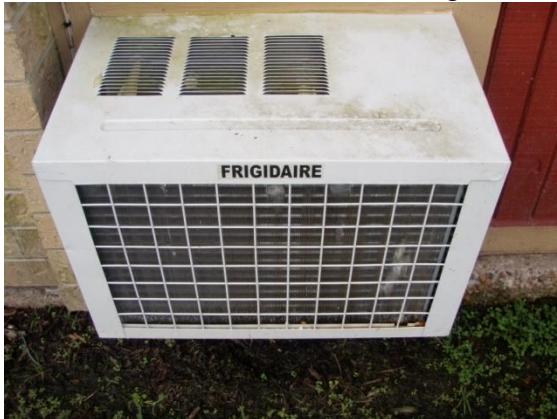
3 Window units for air conditioning.
